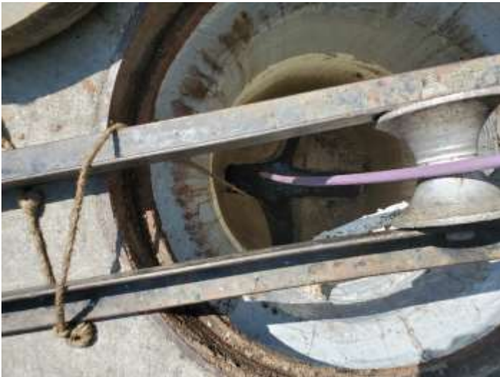
CCTV (St Paul St)
