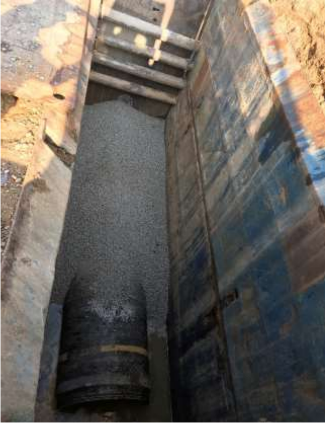
Pressure Sewer (N Broadway)
