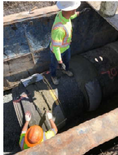
Pressure Sewer (Rutland Ave)
