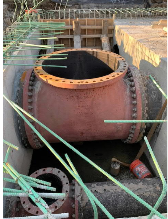
Tee on 54inch Siphon Pipe (Falls Rd)
