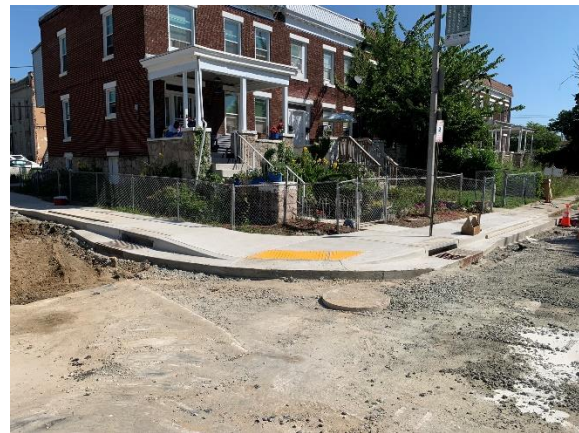
New sidewalks and ramps at Towanda Ave. & W. Cold Spring Ln. (August 2022)
