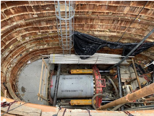
Installation of the final 60" tunnel casing pipe at Daytona Ave & W Cold Spring Ln (Completed April 2022)
