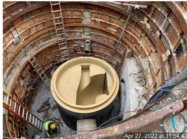
Installation of the 96" diversion manhole at Towanda Ave & W Cold Spring Ln (in-progress)
