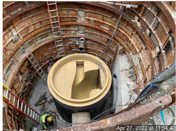
Installation of the 96" diversion manhole at Towanda Ave & W Cold Spring Ln (Completed)
