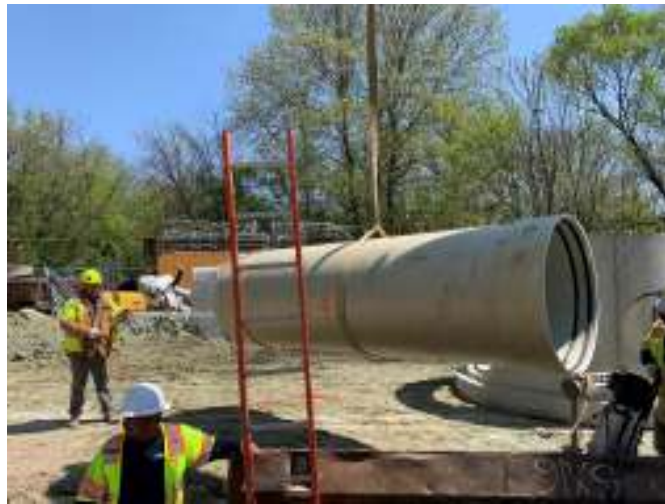
New 42" FRP pipe installation in progress at 2800 N. Dukeland Street (Completed June 2022)
