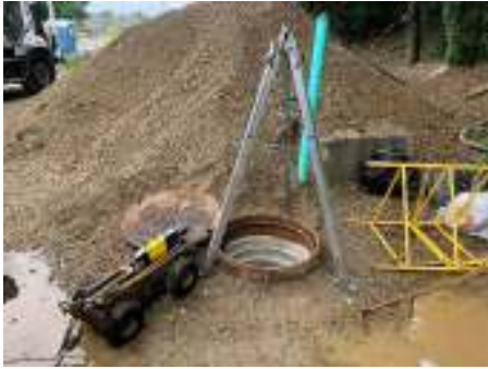
Preparation to Televis (CCTV) the new 42" pipes at 2800 N. Dukeland Street (Completed June 2022)
