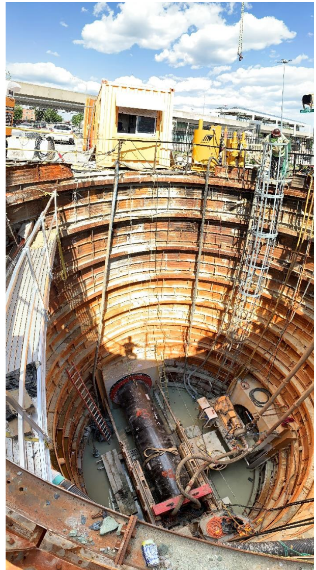
Relief sewer microtunneling underway at the intersection of Wabash Ave & W Cold Spring Ln
