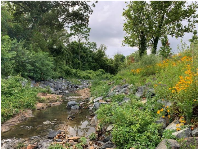
Reach E Stream Restoration Work Complete, new grass and planting installations (between Belvedere & Northern Parkway)
