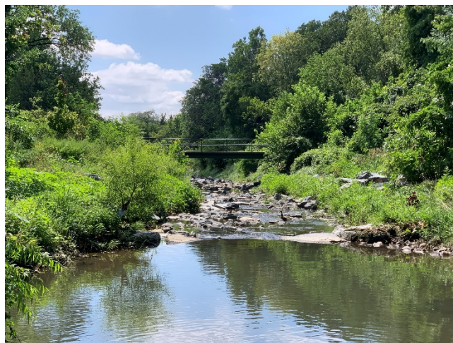
Reach E Stream Restoration Work Complete, Grasses and trees filling in (between Belvedere & The Alameda)
