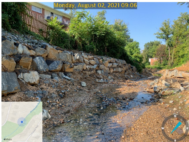
Reach H Stream Restoration Work Complete, Slope stabilization with imbricated rock walls (between Cedarcroft & Walker Ave)
