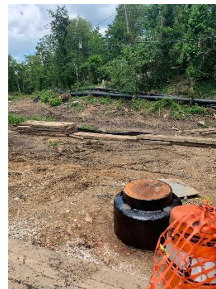
Sewer manhole construction in Reach H (Just upstream of E Lake Ave)
