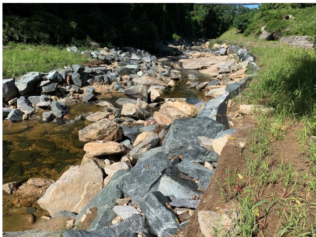
Reach A Stream Restoration Work Complete, Slope stabilization with imbricated rock walls (between Perring Parkway and Herring Run)
