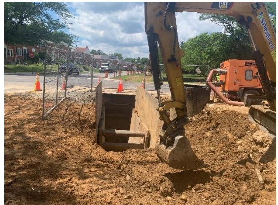
Sewer pipe replacement underway at The Alameda and Northwood Drive, bypass in-place
