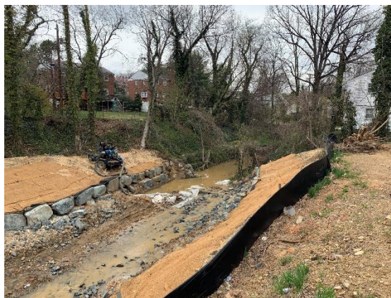
Reach I Stream Restoration Work In-Progress, (between Northern Parkway & E Lake Ave)
