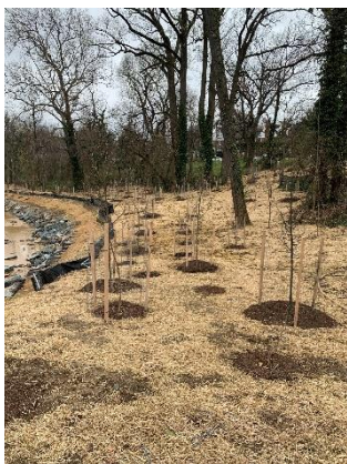
Reach G Stream Restoration Work Complete, new grass and planting installations (between Northern Parkway & E Lake Ave)
