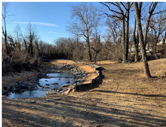
Reach G Stream Restoration Work Complete, ready for future grasses and plantings (between Northern Parkway & E Lake Ave)
