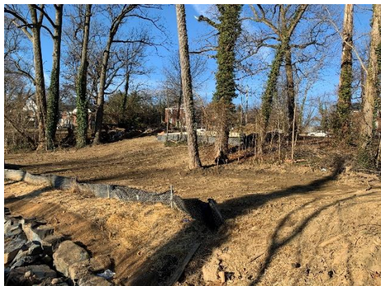
Reach G Stream Restoration Work Complete, ready for future grasses and plantings (between Northern Parkway & E Lake Ave)
