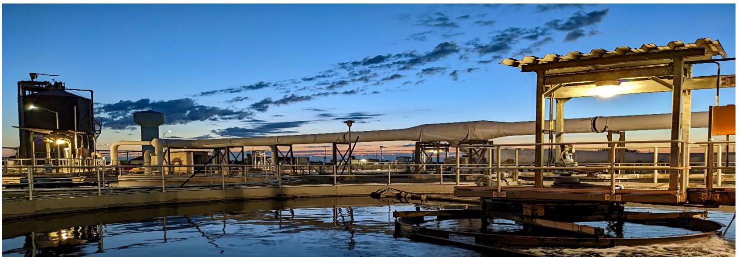
Figure 1: View of Gravity Sludge Thickener
