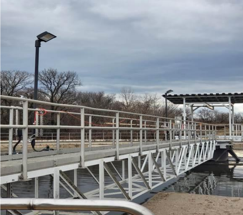
2 New lights installed at the PST Cat Walk at Back River
