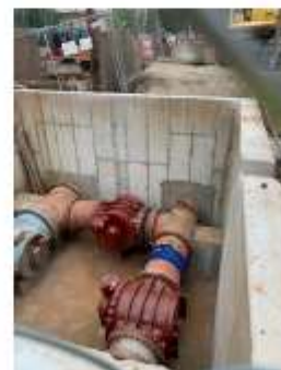
NEW VALVES IN OLIVER ST VAULT
