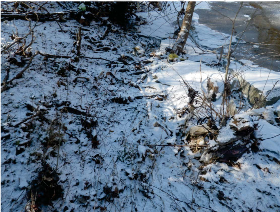
Photo 14. Biddison Run. Scour behind structure vane arm at station 07+40.
