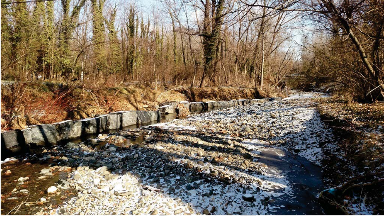
Photo 25. Western Run. Excessive deposition filling the channel and causing left bank lateral erosion.
