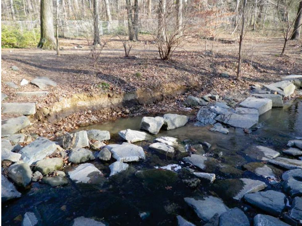
Photo 9. Middle Stony Run. Left bank erosion causing failure of cross vane 6 left vane arm at station 13+35.
