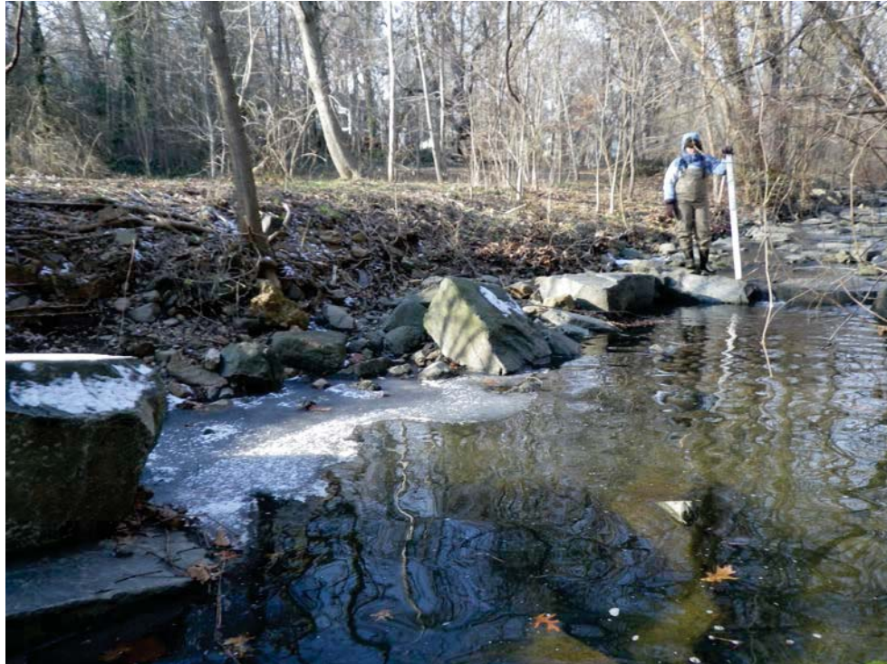
Photo 10. Middle Stony Run. Right bank erosion showing failure of cross vane 7 right vane arm at station 14+30.
