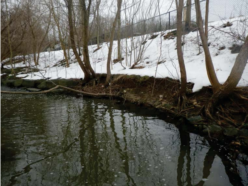
Photo 2. Upper Stony Run. Lateral bank erosion due to improper structure placement at station 25+50.
