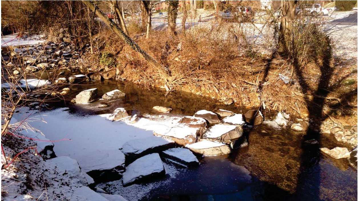
Photo 23. Western Run. Lateral bank erosion causing structure flanking on left bank.
