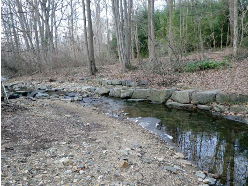
Photo7. Middle Stony Run. Excess sediment causing bar formation and lateral erosion downstream of vane arm at station 10 + 90.
