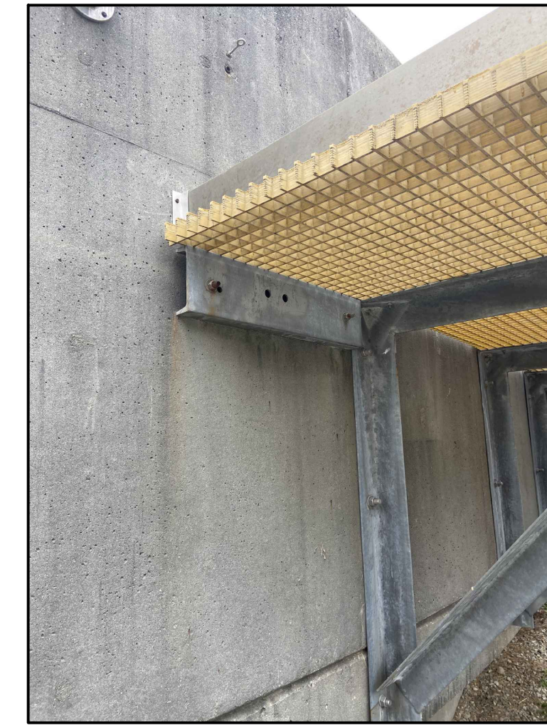
5 PHOTO - CORRODED ANCHORS AT GST WALKWAY S-100-02 SCALE: NTS
