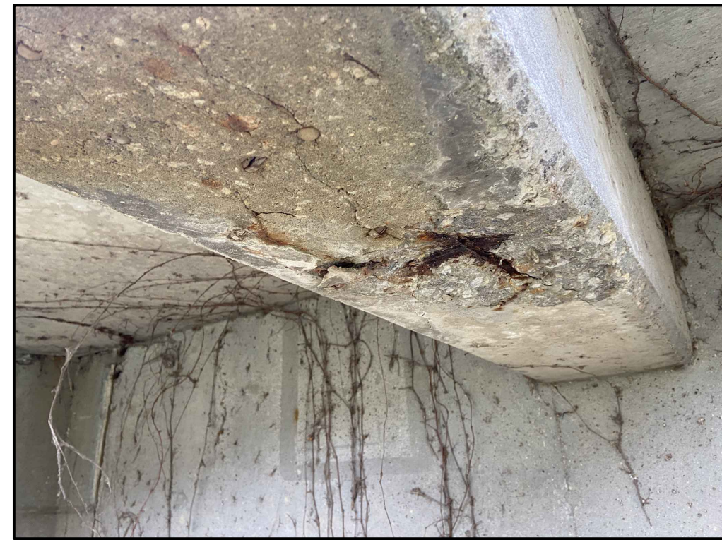
7 PHOTO - SPALL AND CORROSION AT GST EXTERIOR PLATFORM BEAM S-100-02 SCALE: NTS
