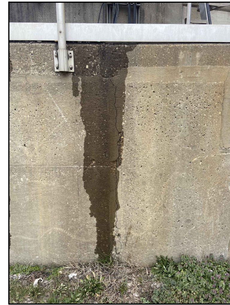
4 PHOTO - CRACK AT GST BUILDING EXTERIOR PLATFORM S-100-02 SCALE: NTS
