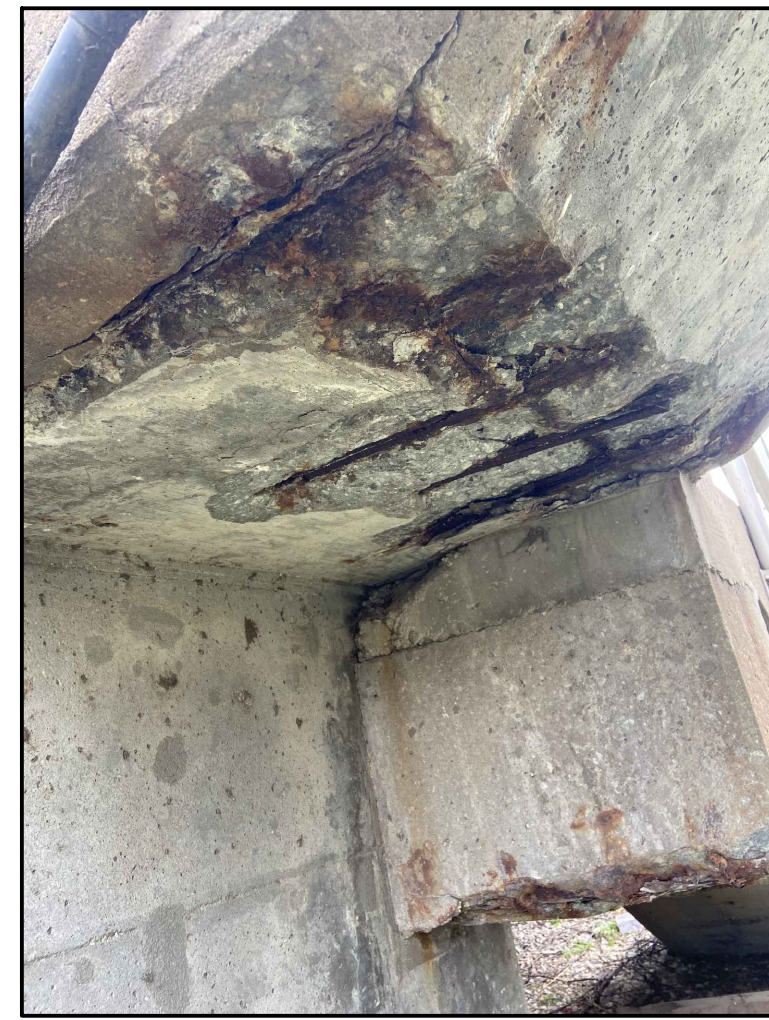
8 PHOTO - SPALL AND CORROSION AT GST EXTERIOR STAIR S-100-02 SCALE: NTS
